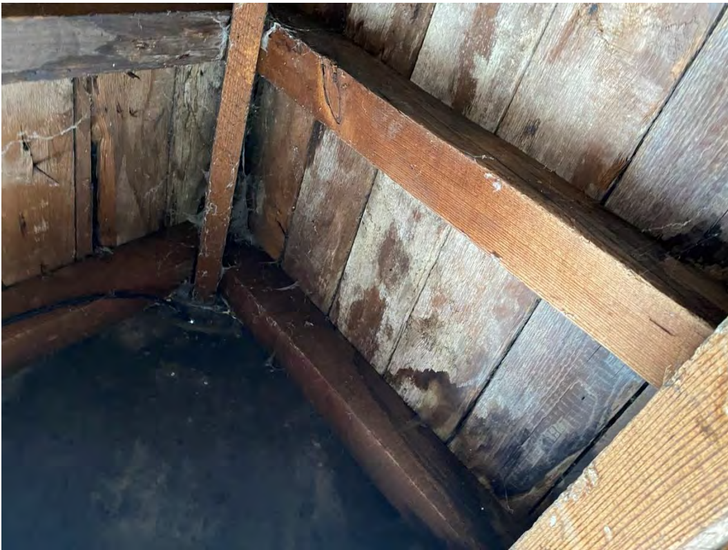
1036) Typical example of moisture stained sarking boards
