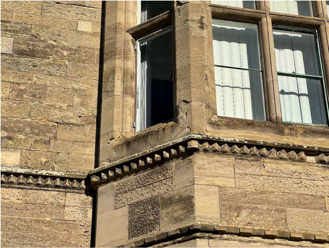
1017) Typical example where replacement stone is required
