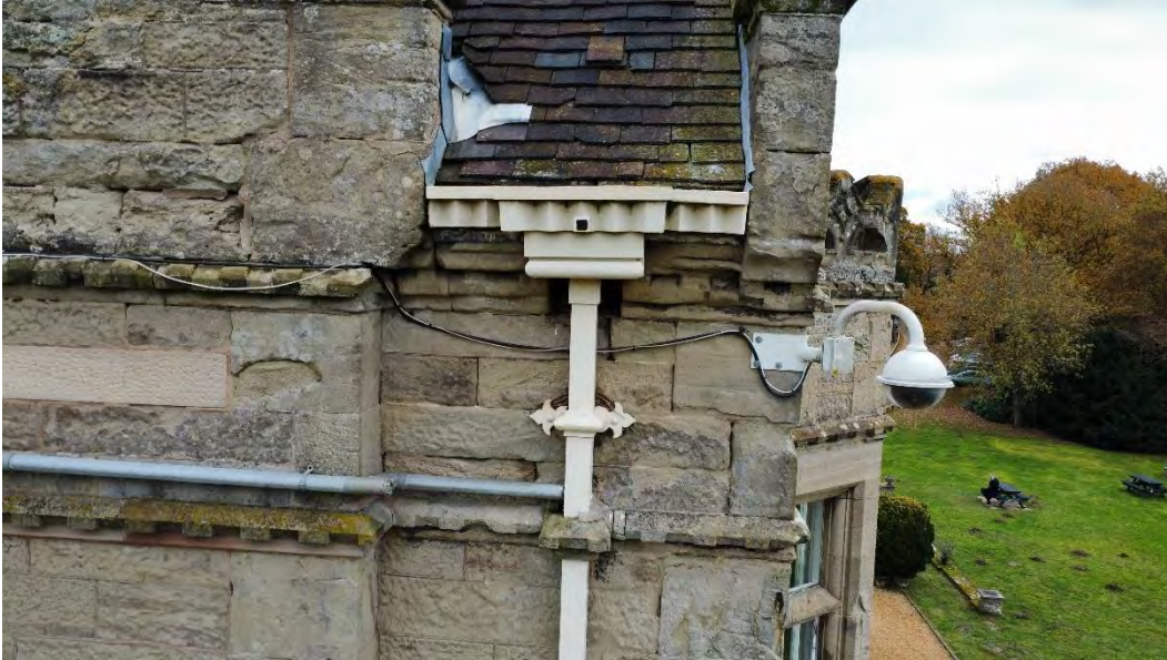
1021) Example where numerous stone defects are present ranging from requiring mortar repairs, armature repairs and replacement stone
