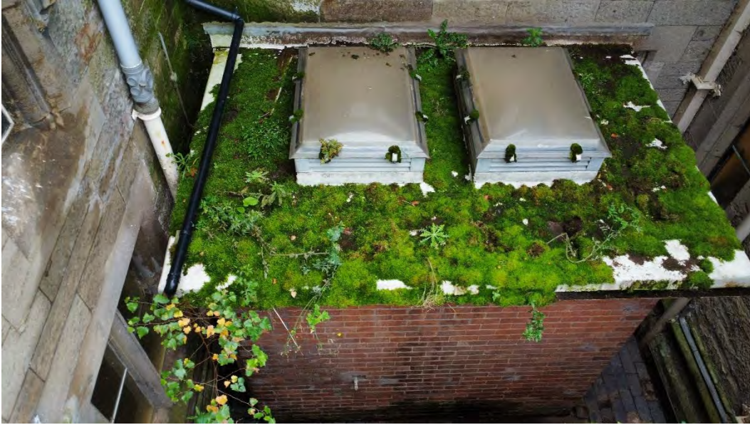
1027) Heavy moss growth to WC roofs
