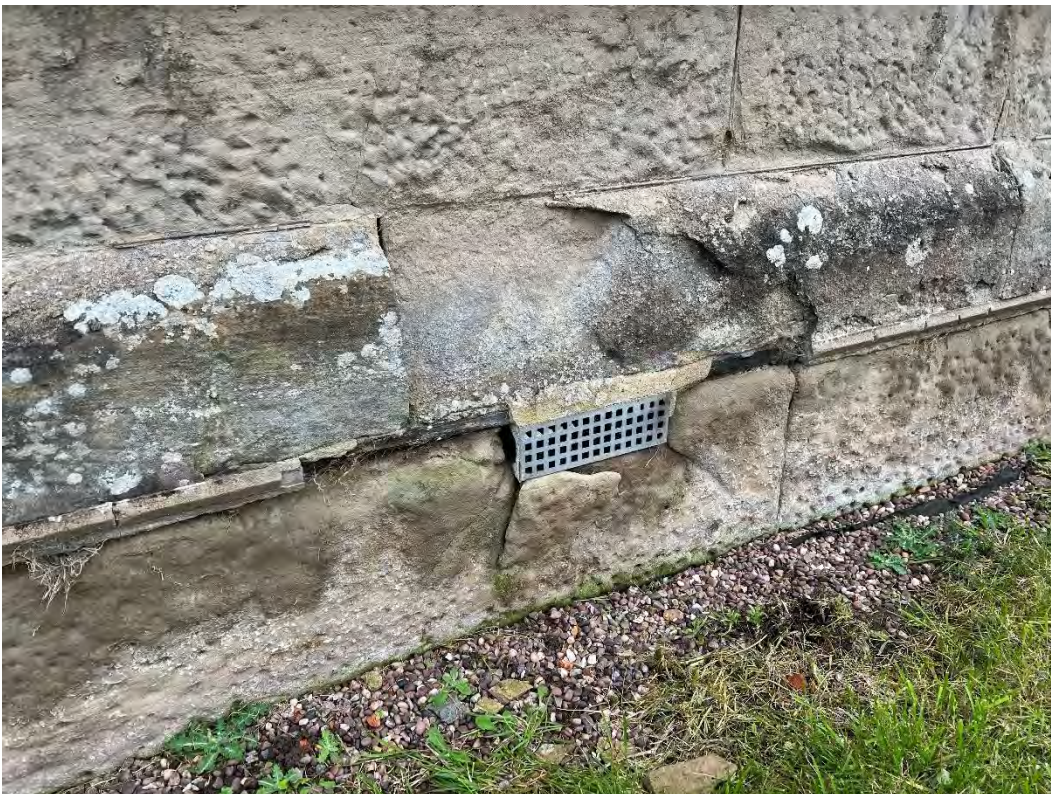
1022) Typical example where replacement stone required
