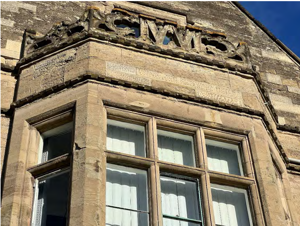
1018) Typical example where partial replacement stone is required
