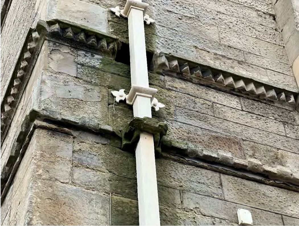
1033) Typical example where string bands are heavily deteriorated and/or missing
