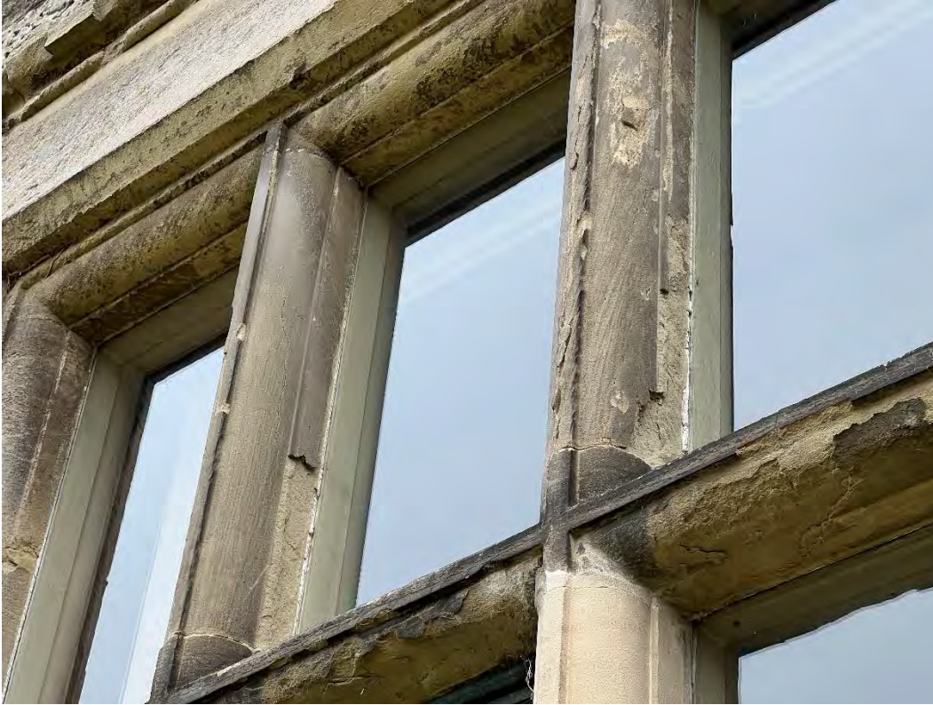
1023) Typical defect to stone window mullions
