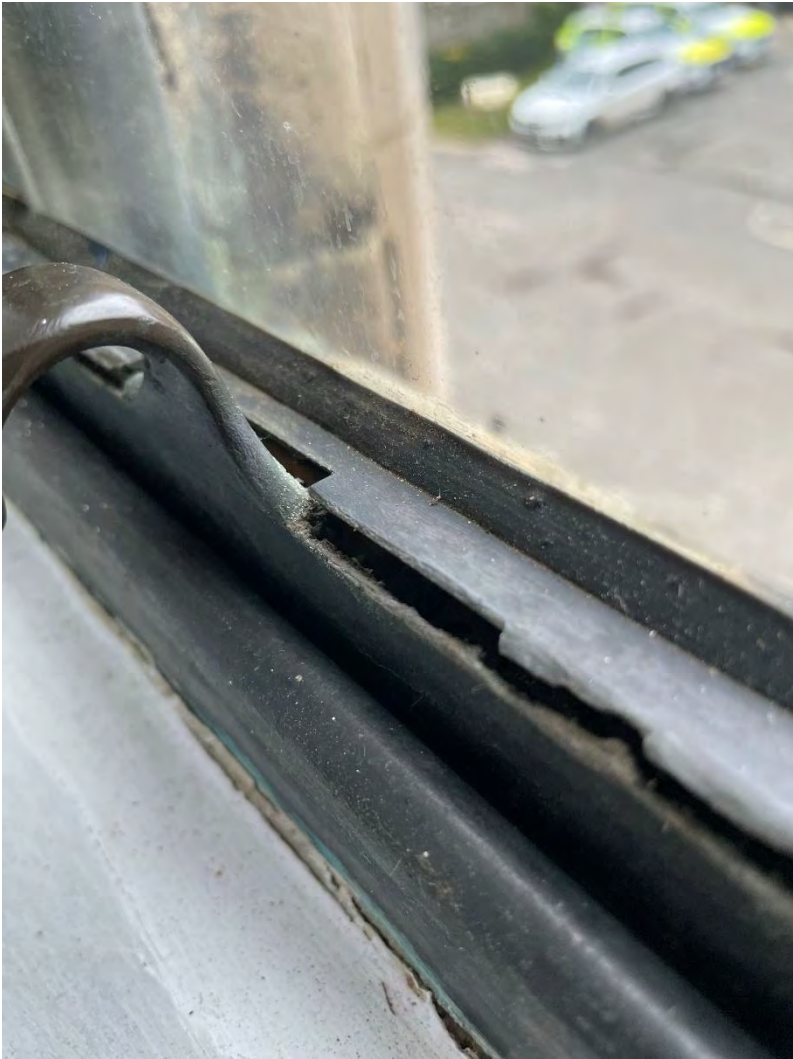
1013) Typical split to metal of sash windows
