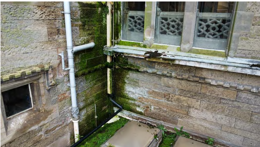
1026) Heavy water damage to stonework with algae and moss growth
