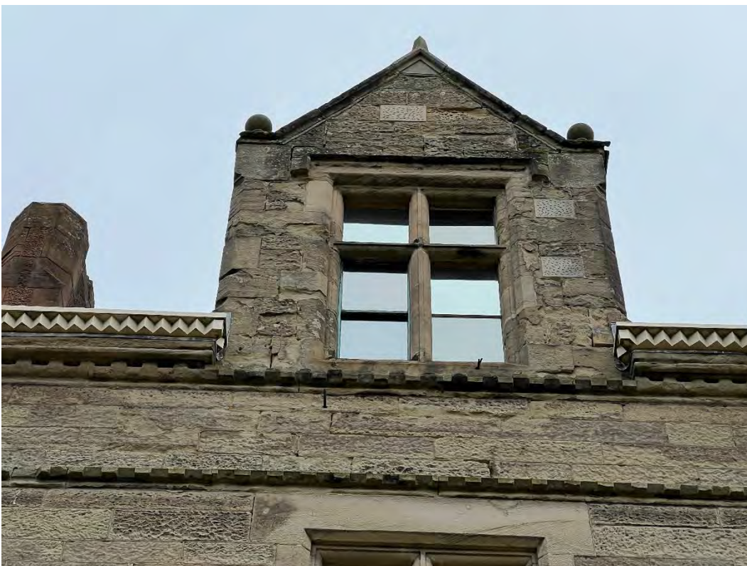
1024) Example where numerous stone defects are present ranging from requiring mortar repairs, armature repairs and replacement stone
