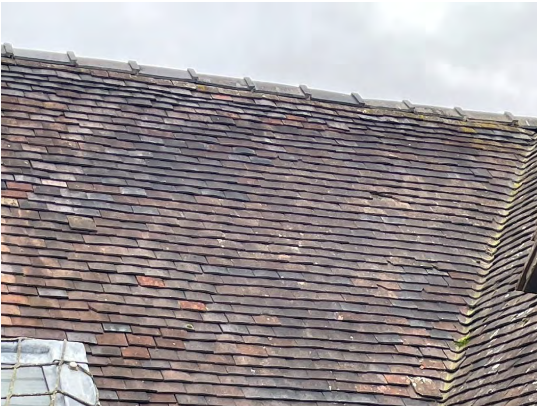
1010) Typical condition of roof pitch – slipped and damaged tiles
