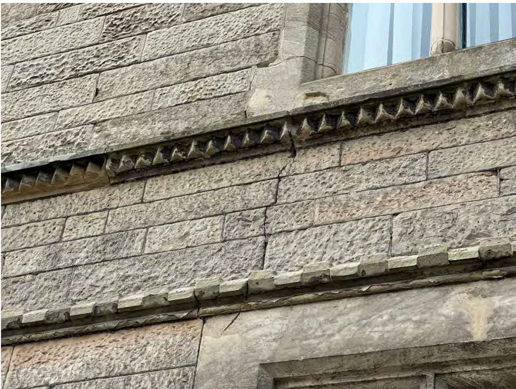
1016) Cracking to Front (East) elevation
