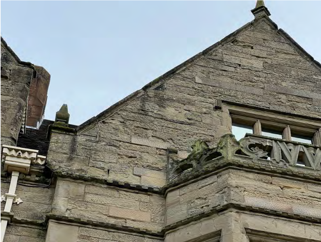
1025) Example where numerous stone defects are present ranging from requiring mortar repairs, armature repairs and replacement stone
