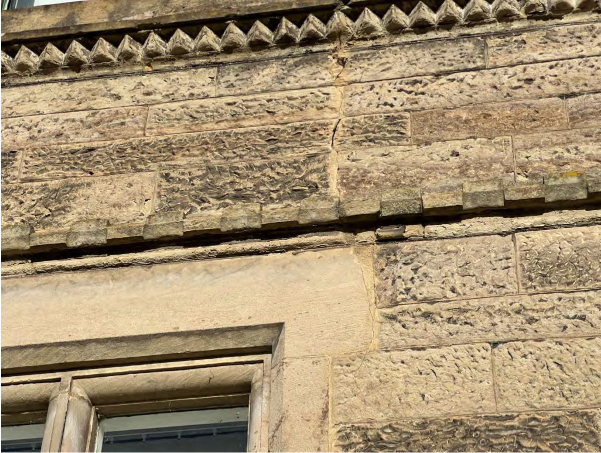
1039) Cracking to left hand side (south) elevation
