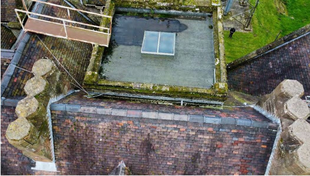
1029) Disconnected leadwork behind flat roof
