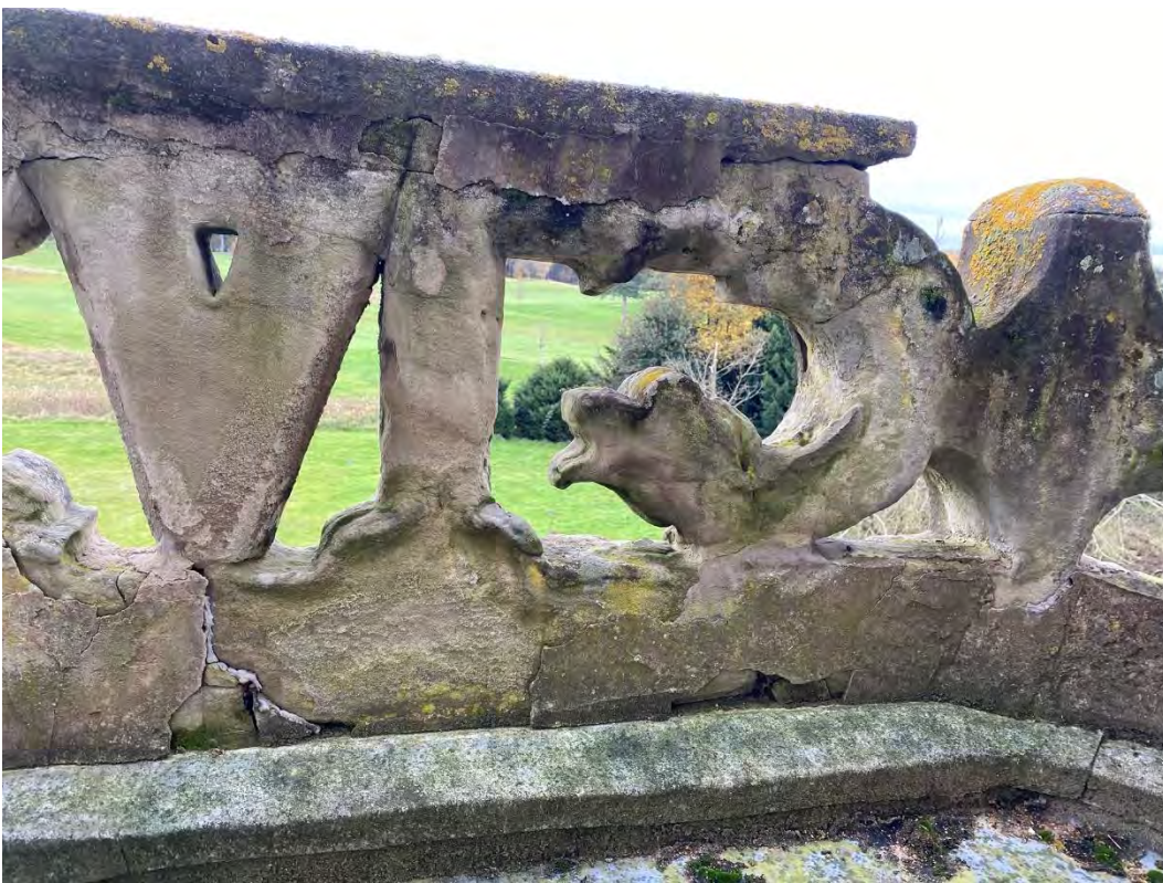
1038) Close up of ornate balustrades in poor condition
