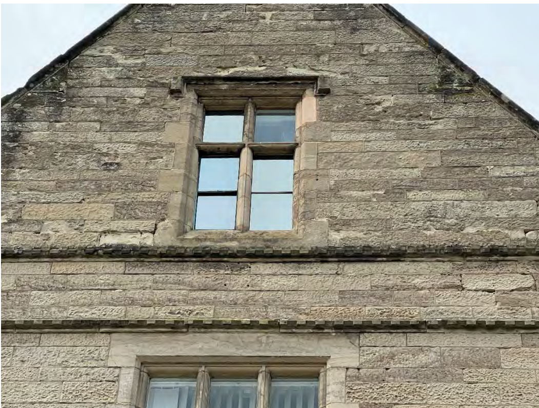
1034) Example where numerous stone defects are present ranging from requiring mortar repairs, armature repairs and replacement stone
