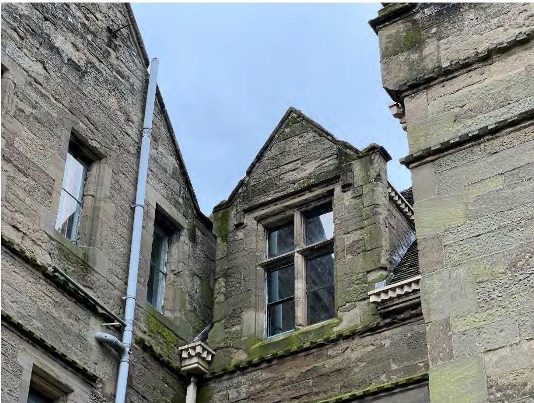
1030) Deteriorated coping stones and missing finials
