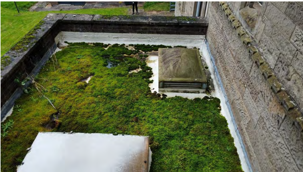
1028) Heavy moss growth to WC roofs – missing flashing to left hand side parapet
